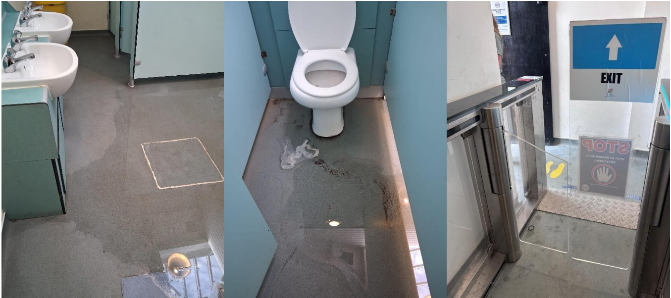
Vandalised and blocked toilets at The Guildhall.
