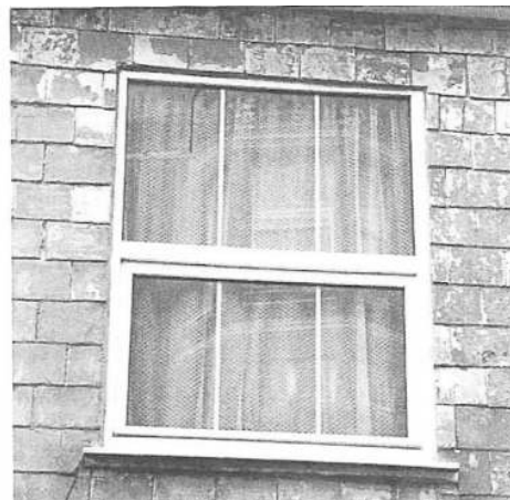
Failed attempt to retain the authentic proportions of an old window. The original pattern of the above example can only be surmised!
