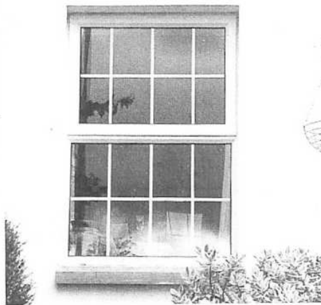
Compare this with the original window shown adjacent. The 'meeting rail' is the widest element, while the bottom of the lower sash is the thinnest! These subtle changes in detailing spoil the proportions.
