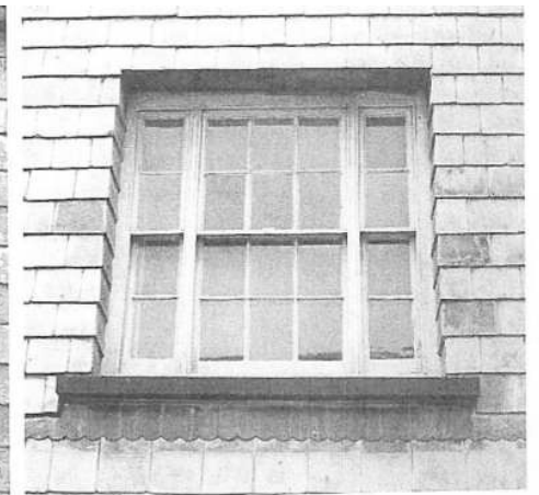
The original method of glazing a square proportioned opening. Note that the vertical proportions are retained by subdivision into smaller sliding sash windows. Avoid the use of decorative lead flashing on older properties.
