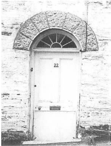
Retain and repair original joinery. Note the fan light is positioned over the door, and the correctly detailed glazing pattern. Repairing this door would be cost-effective in comparison to replacing it with a new one.
