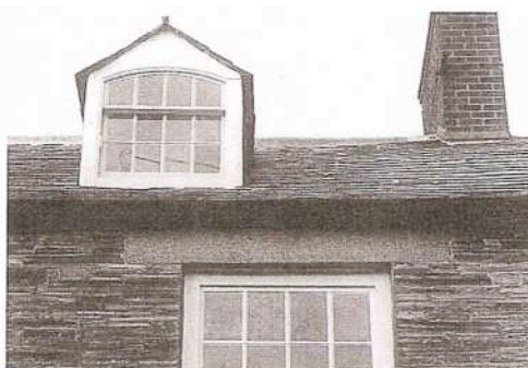
Pitched' dormers are the most typical in the area but are more complicated to construct. Note the small scale of the dormer compared to the window on the main facade. Lead or slate are suitable materials for the dormer cheeks.
