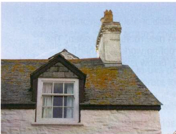
Fig 19: An attractively detailed eaves dormer is a later addition. Note the absence of guttering and simple moulded edges to fascia and barge boards
