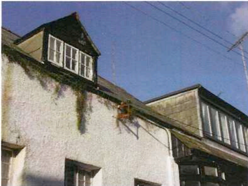
Fig 15: If gutters are not cleared of debris plants soon take over and the rainwater spills over the face of the building [see also Fig 20]
