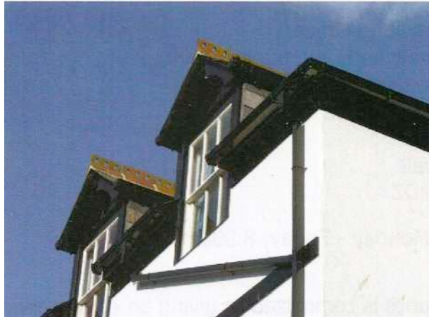
Fig 21: This plastic ogee guttering is not even close to the elegance of the historic version; the unnecessarily complicated down pipes in box profile are an unattractive addition
