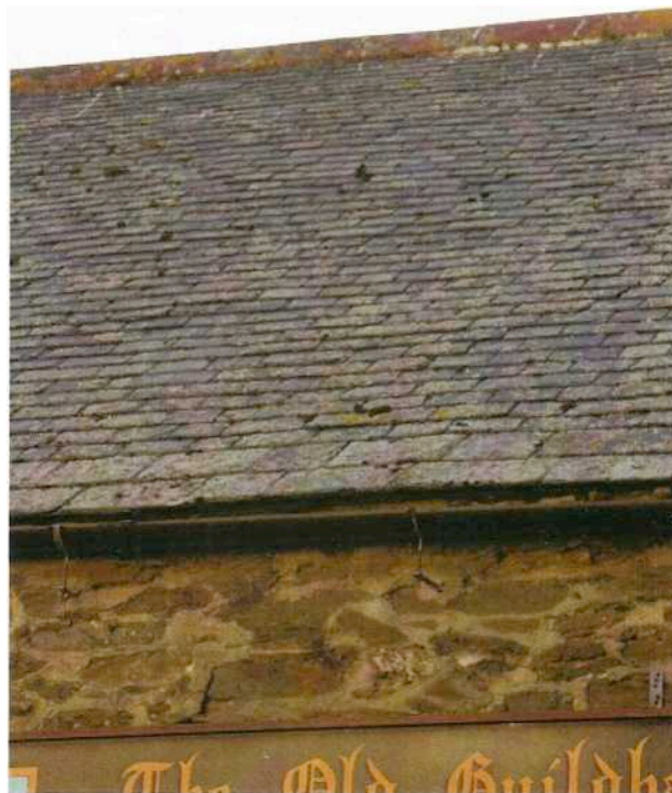
Fig 3: Traditional roof on the Old Guildhall with slate laid in diminishing courses
