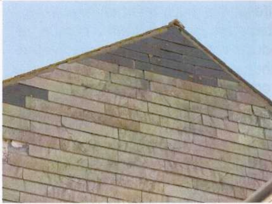
Fig 12: A simple mortar fillet between the roof and rag slated gable end (note that slate is hung back-to-front to give a natural drip)
