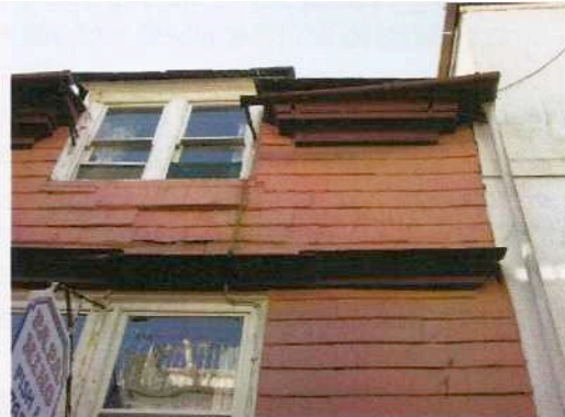
Fig 16: This broken gutter fixing has clearly been discharging water onto a very important historic facade for some time. It is causing costly damage to slate hanging, cornice and probably structure; it is also a potential danger to pedestrians below
