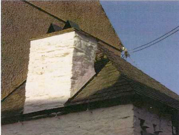
Fig 8: Half round cast iron guttering fixed using spiked brackets, so avoiding the need for a fascia board
