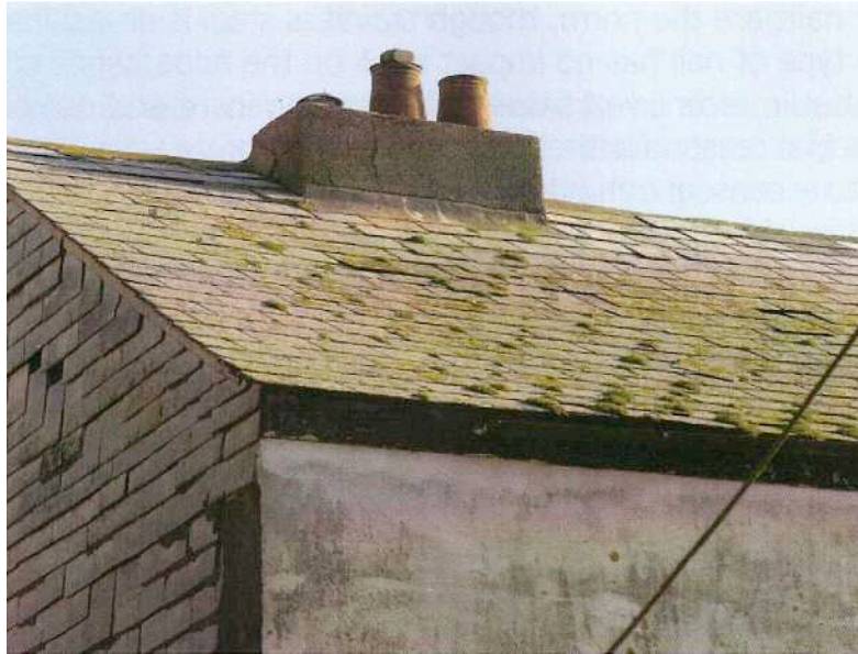
Fig 5: Sized Delabole slates with slippage due to nail rot .many of the slates could be re-fixed though
