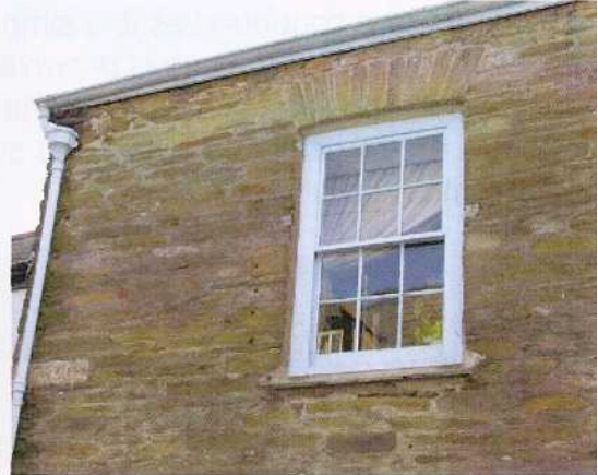
Fig 9: Ogee cast iron guttering fixed to a shallow fascia with no overhang or soffit
